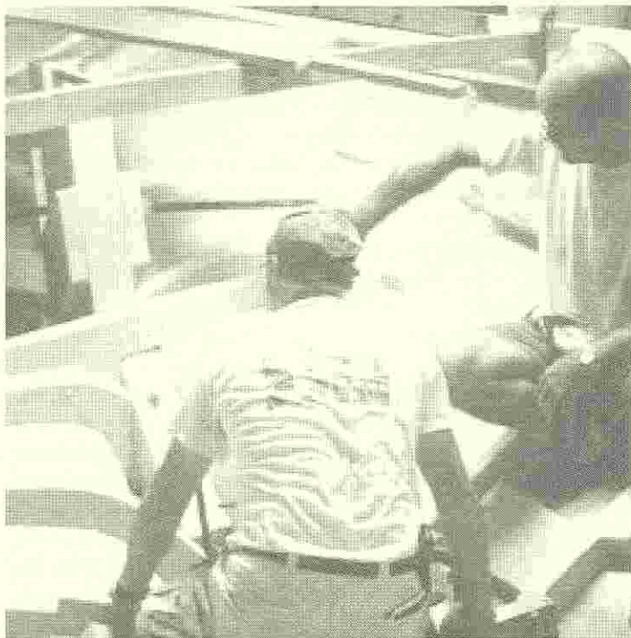
Figure 2. Rick and Graham discussing alignment of drilling jig. Graham's right hand rests on one of the vee blocks. (Photo by Brian McCandless)
